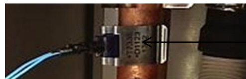
Heating Sensor Secured With Spring Clip to Pipe
